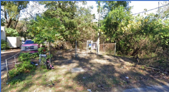
Hilly Road Pump Station
