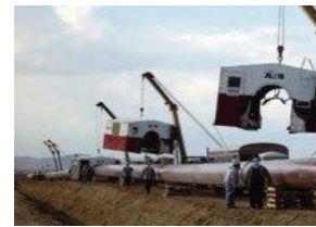
Kern River Pipeline
