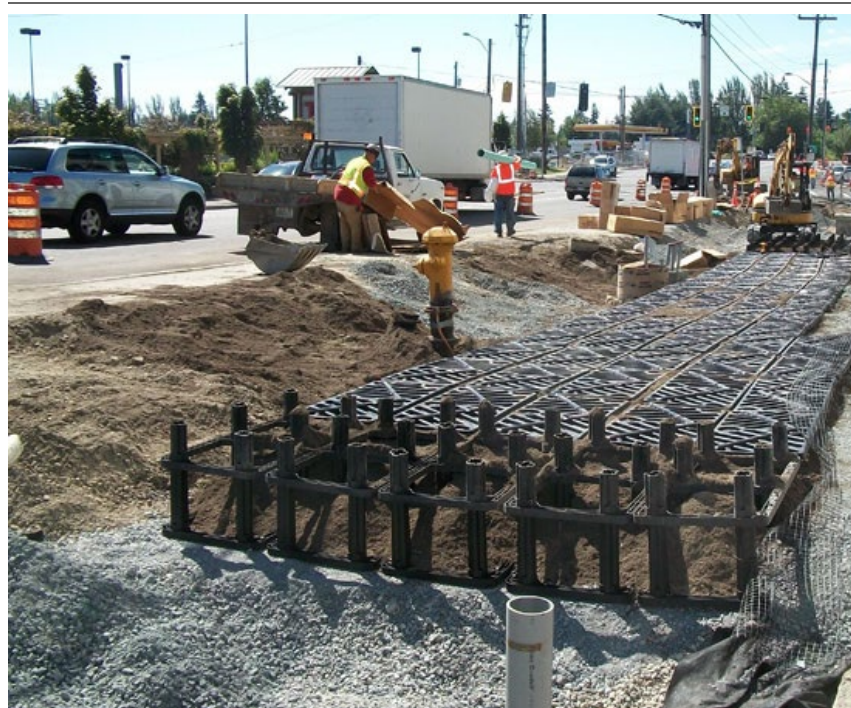
The Aurora Avenue streetscape project in Seattle, Washington during the installation of a soil cell system.
