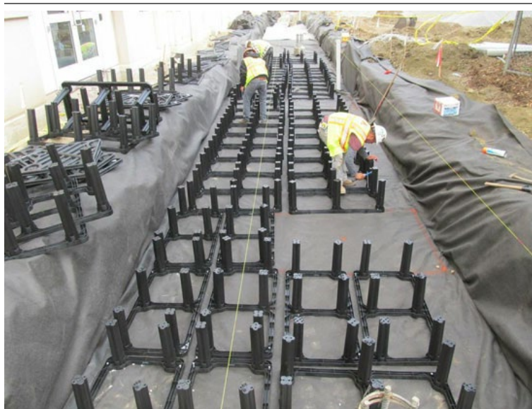
A soil cell system was used to meet new storm water runoff requirements at a courtyard project in Menlo Park, California.
