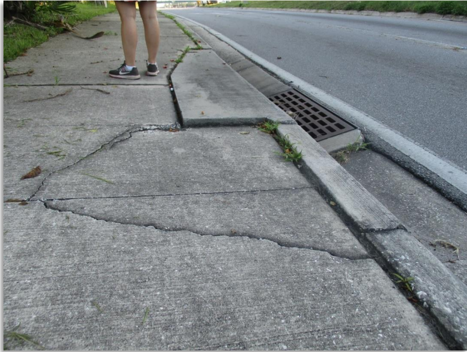
Figure 6: Severely broken sidewalk with no grassed buffer
