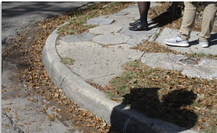
Figure 5: Broken sidewalk with no curb ramp
