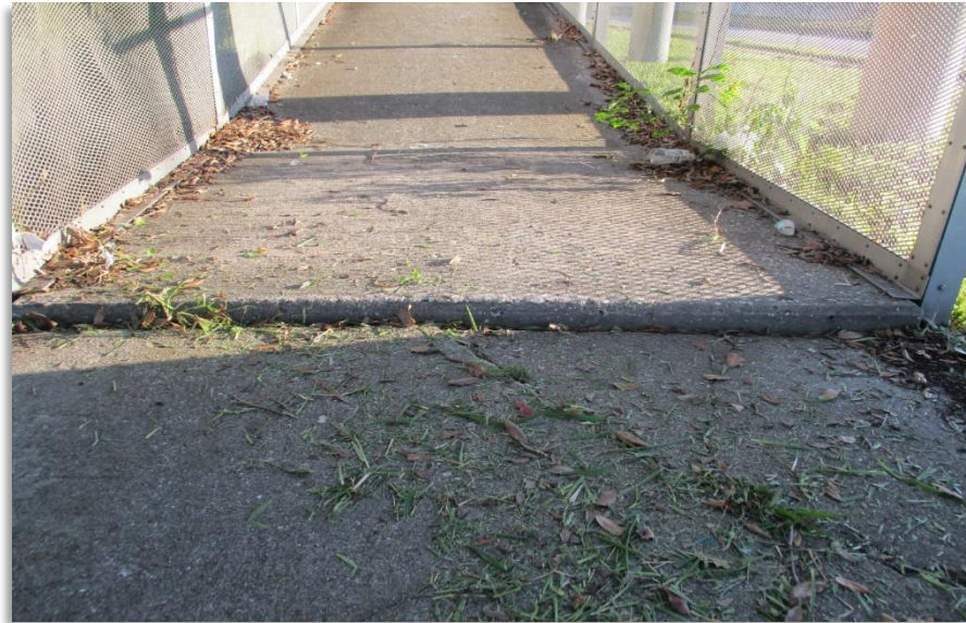
Figure 16: Broken sidewalk on pedestrian overpass at Haines Street and Winthrop Street
